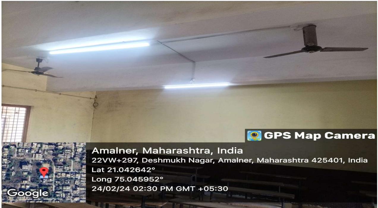
LED Light Use In Classrooms
